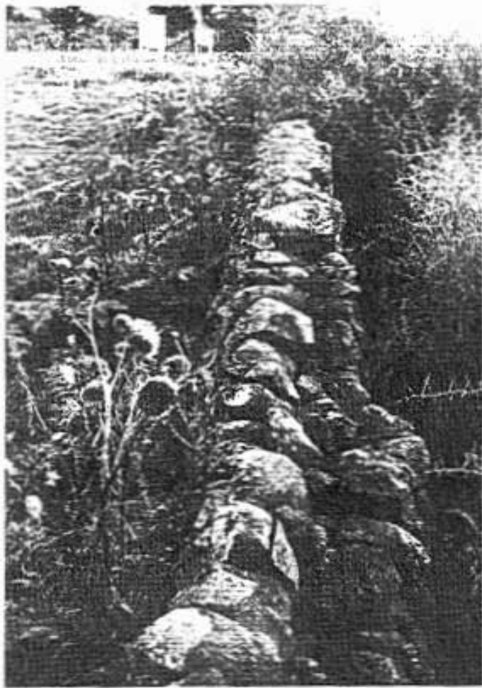
Site No. 014 Detail of Wall Construction Note Missing Cope
