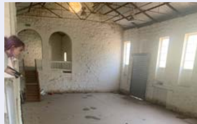
The waters receded in the historic Bluestone Building leaving behind a thin layer of mud.
