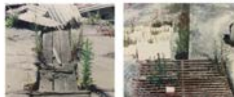
Images below (1997) methods of covering drains and drains used to inform the 1998 works. The timber slab method was used in many locations.
